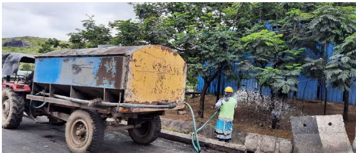
Permeate used to maintain greenery in the site
