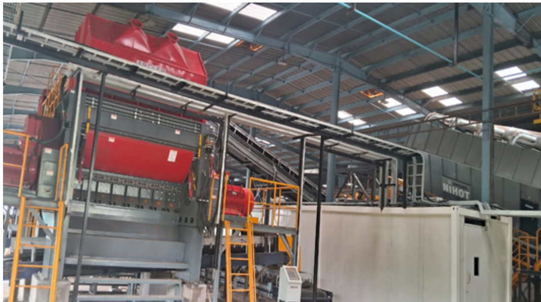
RDF manufacturing unit
