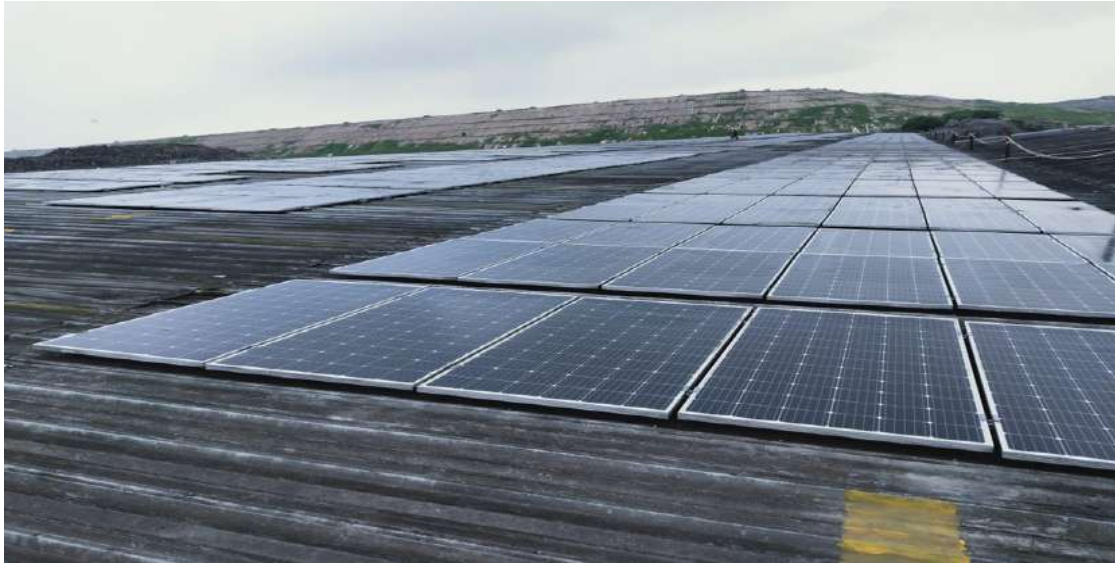
1MW solar energy plant
